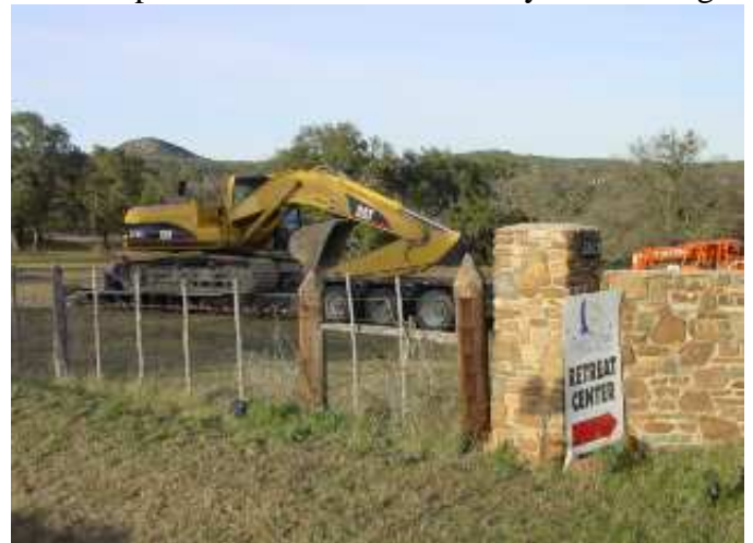
Matous Construction delivering heavy equipment to start on Waste Water Treatment Plant
